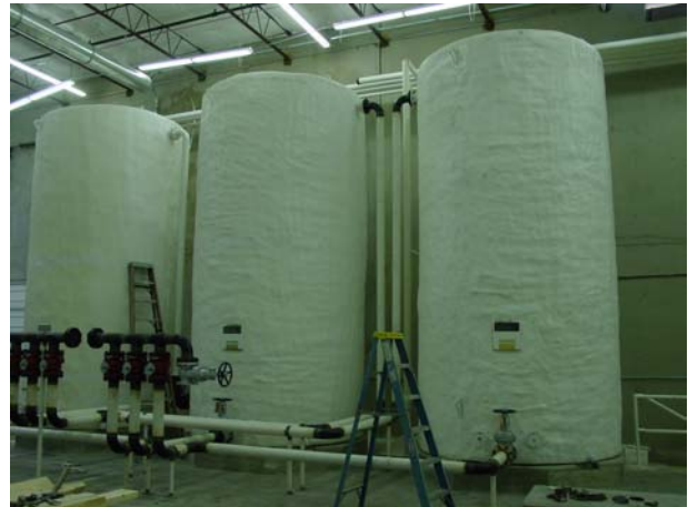
Three 6,000 gallon heated and insulated chemical tanks. Tanks, pumps, meters and piping installation by Smith Tank.
