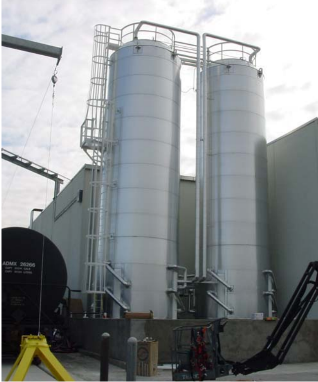
Two 27,000 gallon heated, insulated and jacketed tanks for liquid food products.
