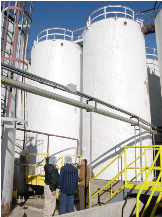
Two 30,000 gallon heated/insulated vegetable oil tanks with handrails and cross walks.
